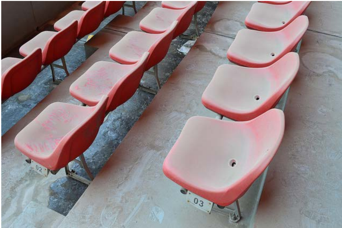
Figure 45: Red Lantern Stadium seats. The seats were covered in a thick layer of dust, either from lack of use, pollution, or both. Site visit, 2014.
