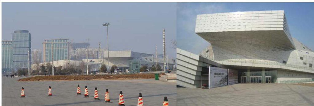
Figure 38: Taiyuan Museum of Fine Arts. Meant to be bright white, the building is already discolored and on some sides, missing tiles. Site visit, 2014.
